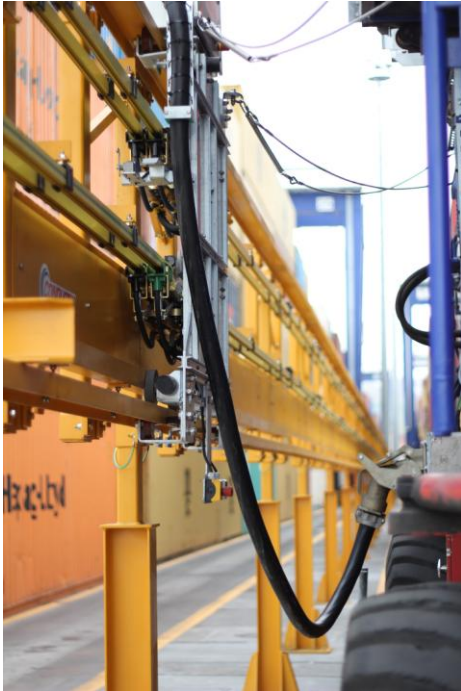
Caption: The plug-in solution from Conductix-Wampfler in use at Marport near Istanbul
