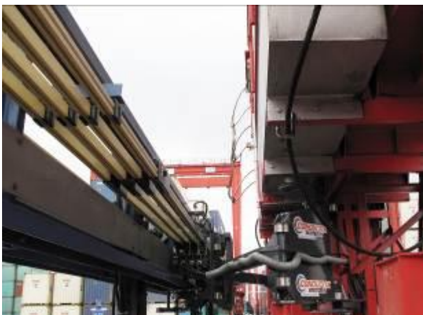
Caption: Since 2009, E-RTGs equipped with the “drive-in” system have been moving about the container corridors of the Shekou Container Terminal in China
